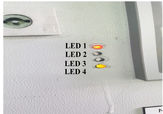
Fig. 6 LEDs for checking operation of sludge monitoring system
